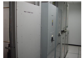
Power Filtering & Switching
