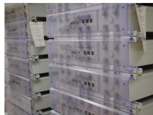
UPS Battery Backup
