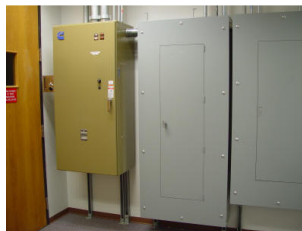
Generator control & switching
